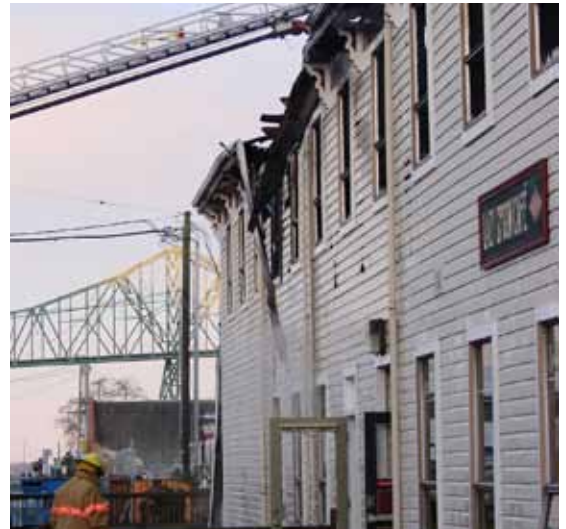
Firefighters assess the damage at No. 10 Sixth Street in Astoria after a fire destroyed the building December 16. Clatsop Behavioral Health, an OHN provider site, was one of 27 businesses lost along the waterfront. (Photo courtesy of Coast River Business Journal).
